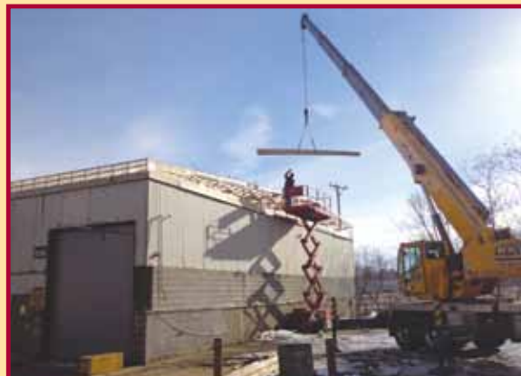
FM Construction recently added a new pitched roof to the Joy Winch building in Buchanan, MI.
